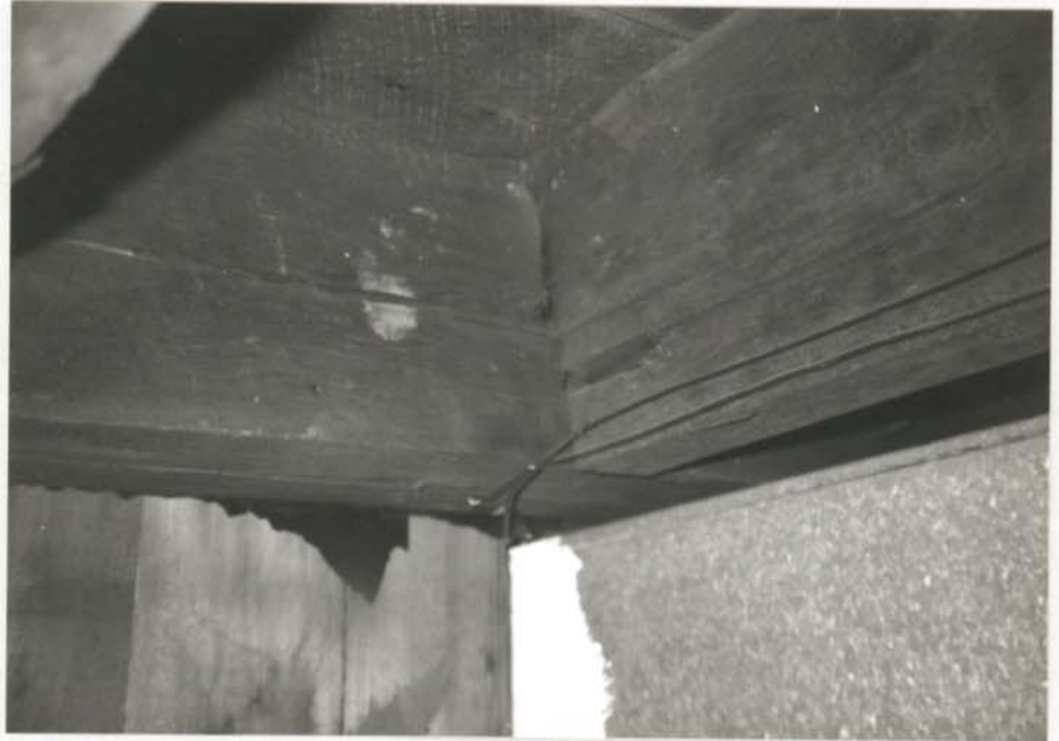
Typical joist-beam detail showing notched joists and splitting beams and joists. This presents a potential structural and safety problem.
