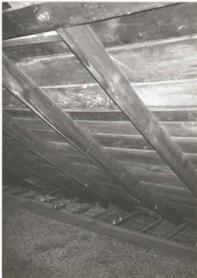
Inside attic the rafters are 2 x 6's and 2 x 4's with significant bowing. Heavy snow loading could cause collapse. Also note: post and tube electrical which is not allowed under today's electrical codes. Home already has had one fire in it in past years.
