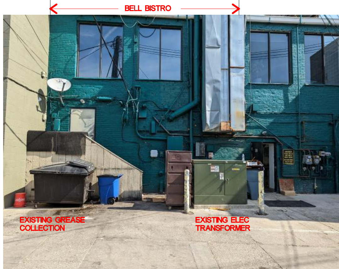
Image B - Rear Alley | Transformer/Utilities
