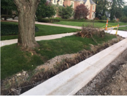
Tree Root Debris on Tilbury Street, 6-30-24..JPG 165K
