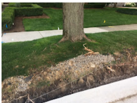
Tree Root Damage on Tilbury Street, 6-30-24...JPG 163K
