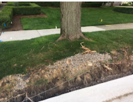
Tree Root Damage on Tilbury Street, 6-30-24..JPG 163K
