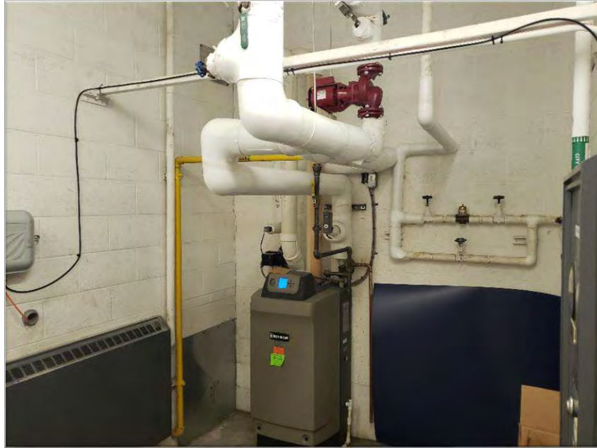
Interior mechanical room
