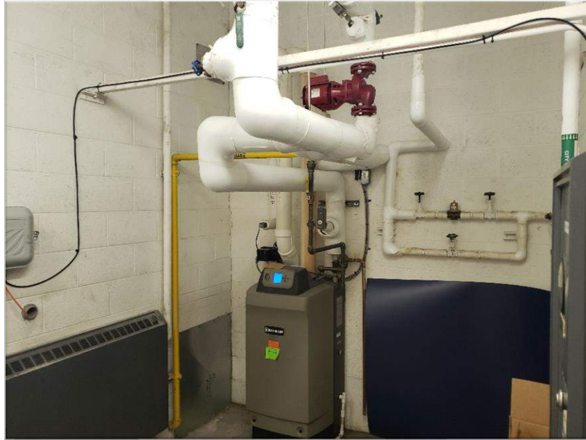
Interior mechanical room
