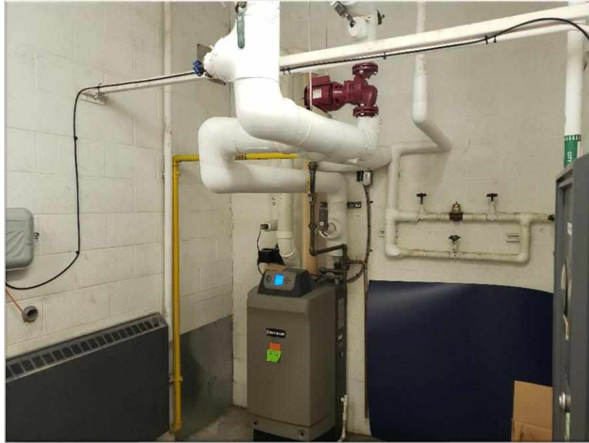
Interior mechanical room
