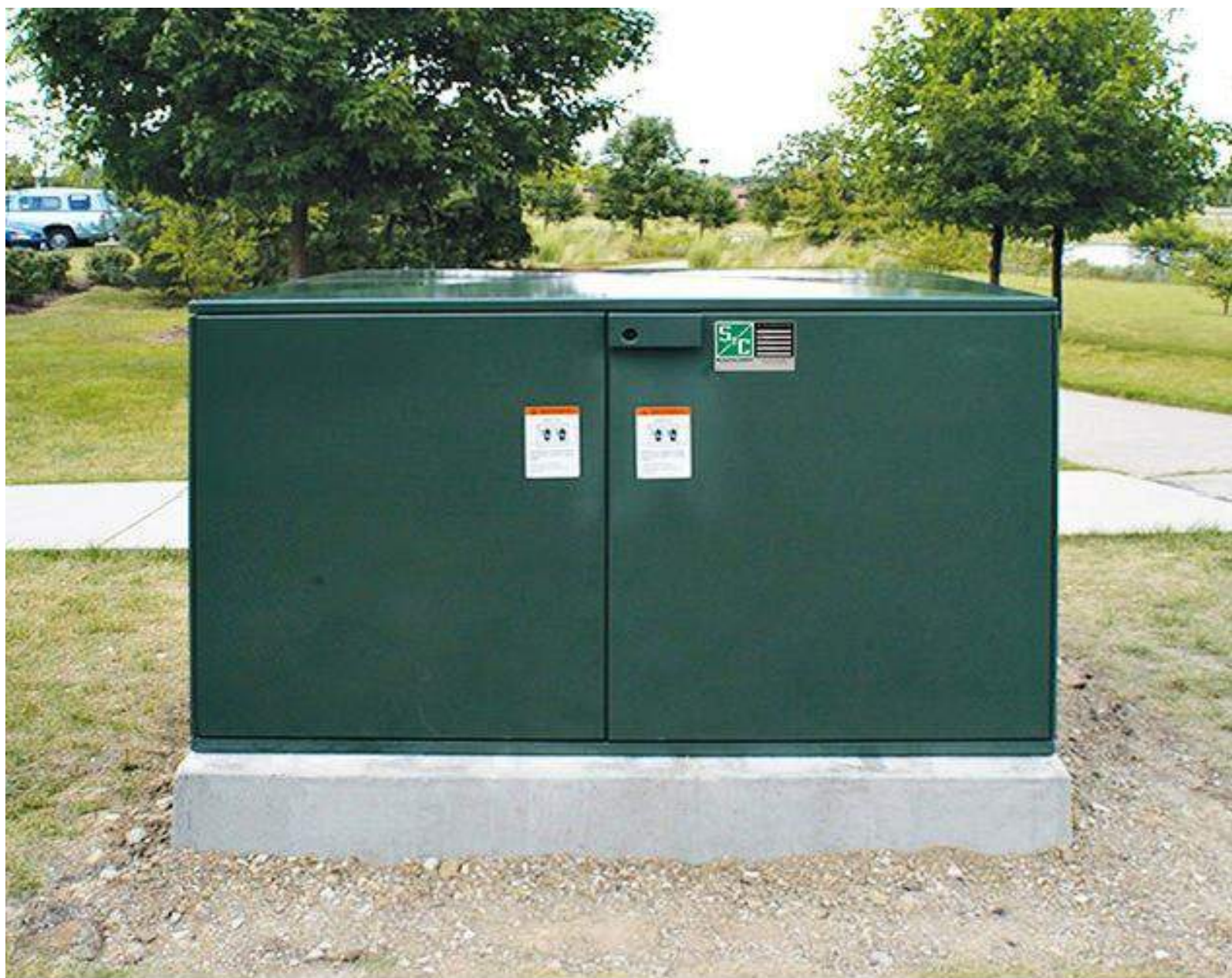
DTE PRIMARY SWITCH PAD IS APPROXIMATELY 36" WIDE BY 44" DEEP. SWITCH IS ABOUT 44" HIGH.
