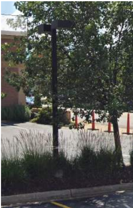
EXISTING LIGHT POLE FIXTURE - TYPE B
