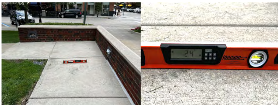
IMAGES 4.1.33 - ACCESSIBLE ROUTE CROSS SLOPE 2.4% > 2%
