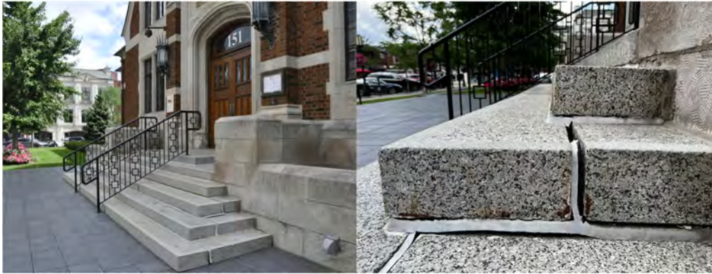
IMAGES 3.1.03 CAULK AT STONE STEPS FAILING
