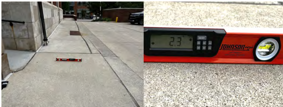
IMAGES 4.1.36 - RAMP LANDING SLOPE 2.3% > 2%.
