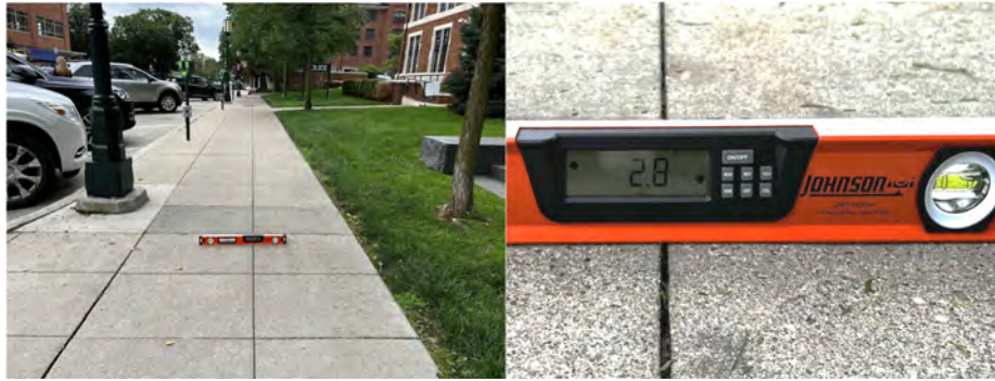
IMAGES 4.1.23 - ACCESSIBLE ROUTE CROSS SLOPE 2.8% > 2%
