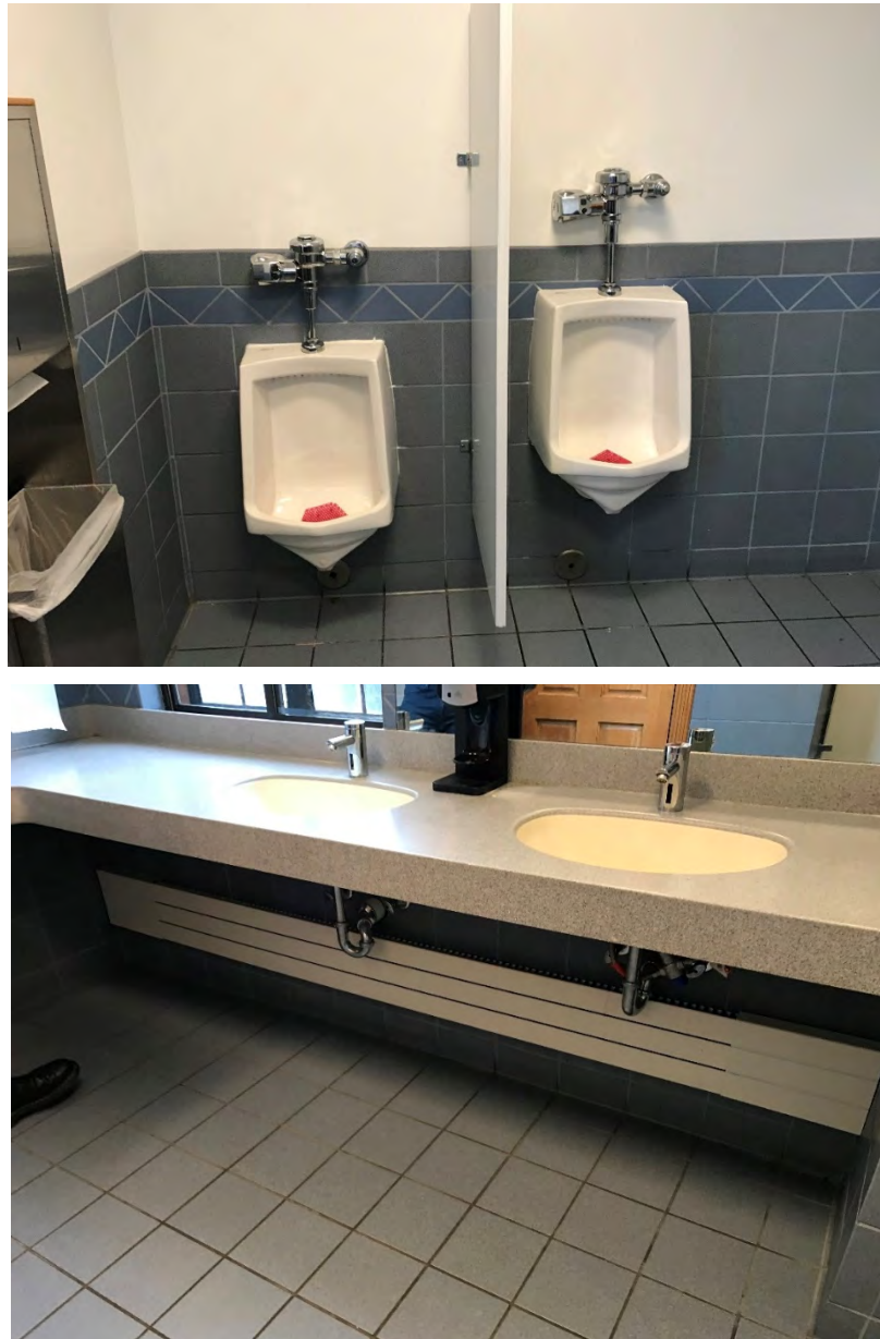
IMAGE 6.19 - RESTROOM PLUMBING FIXTURES
