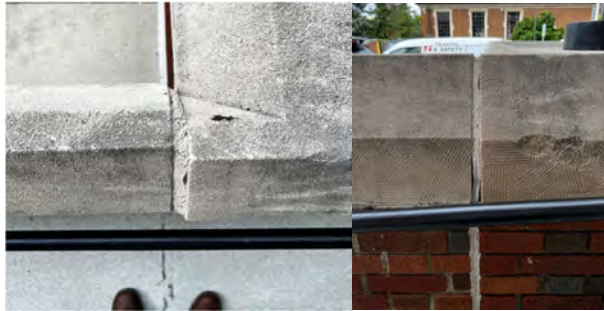
IMAGES 4.1.46 - POLICE DEPT RAMP HANDRAIL GRIP OBSTRUCTION
