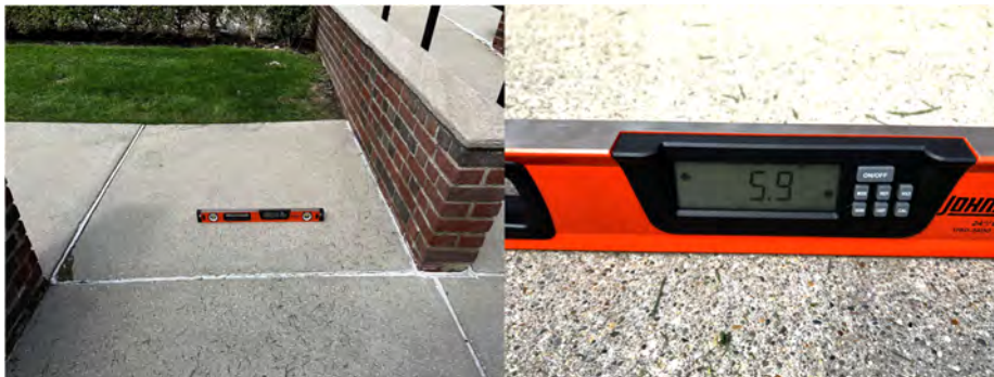
IMAGES 4.1.31 - ACCESSIBLE ROUTE CROSS SLOPE 5.9% > 2%
