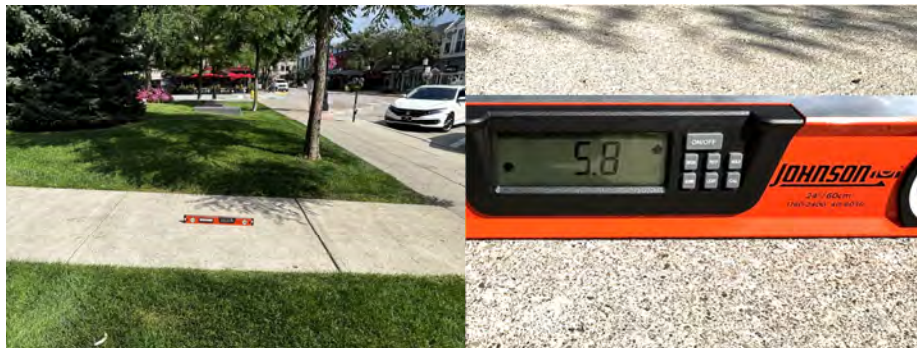
IMAGES 4.1.24 - ACCESSIBLE ROUTE RUN SLOPE 5.8% > 5%
