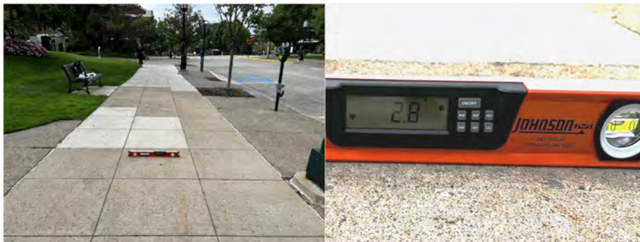
IMAGES 4.1.17 - ACCESSIBLE ROUTE CROSS SLOPE 2.8% > 2%
