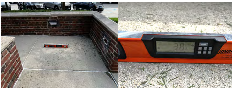
IMAGES 4.1.29 - RAMP LANDING SLOPE 3.8% > 2%
