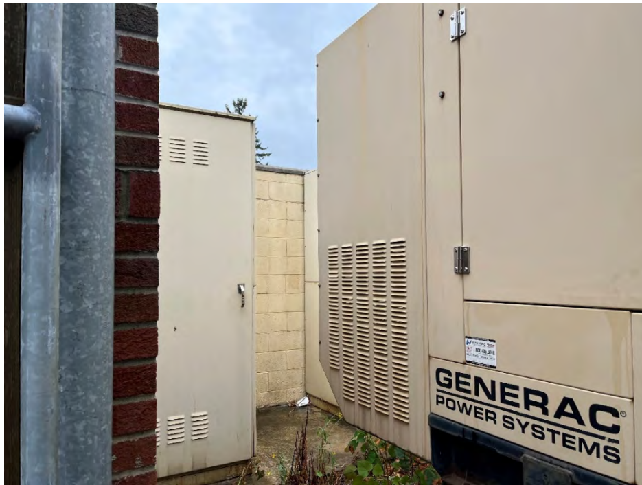
IMAGES 7.4 - EMERGENCY AND STANDBY POWER
