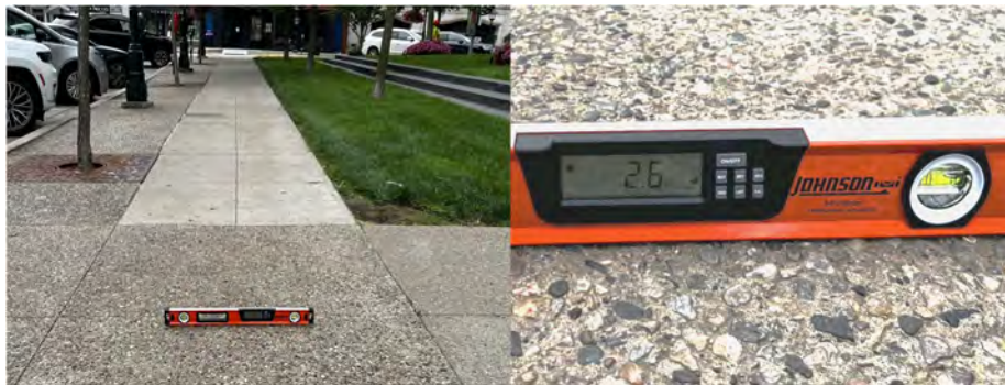
IMAGES 4.1.20 - ACCESSIBLE ROUTE CROSS SLOPE 2.6% > 2%
