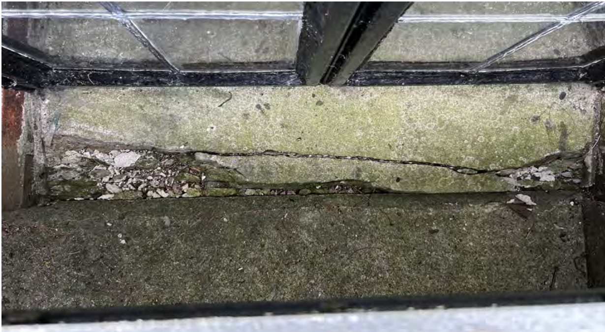
IMAGES 3.1.17 CRACKED CONCRETE SILL
