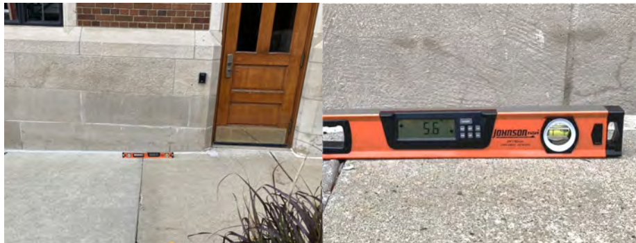
IMAGE 4.1.16 - ACCESSIBLE ROUTE RUN SLOPE 5.6% > 5%
