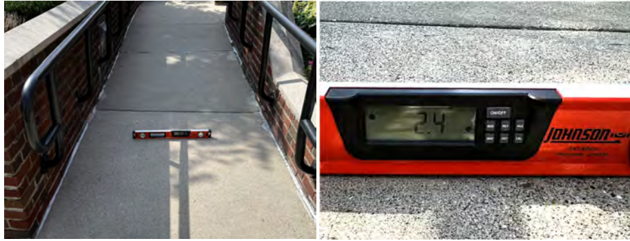
IMAGES 4.1.27 - RAMP LANDING SLOPE 2.4% > 2%
