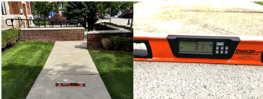
IMAGES 4.1.32 - ACCESSIBLE ROUTE CROSS SLOPE 3.1% > 2%
