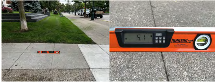
IMAGES 4.1.19 - ACCESSIBLE ROUTE CROSS SLOPE 5.1% > 5%
