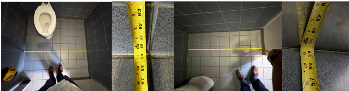
IMAGE 4.2.33 - 1ST FLOOR MENS WATER CLOSET CLEARANCE
