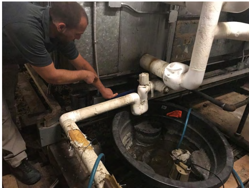
IMAGES 6.9 - HVAC MULTIZONE UNIT
