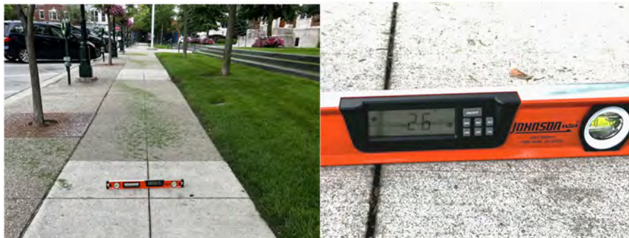
IMAGES 4.1.21 - ACCESSIBLE ROUTE CROSS SLOPE 2.6% > 2%
