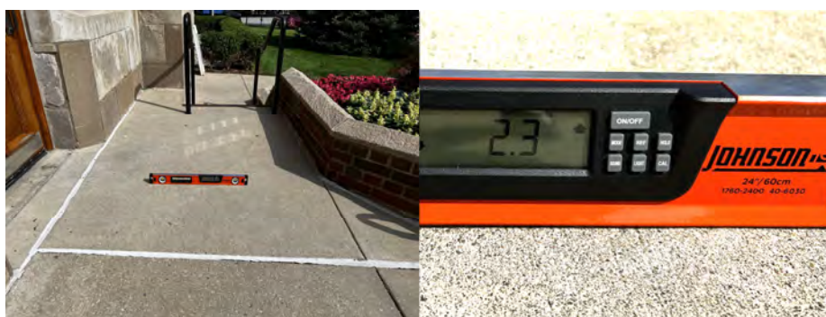
IMAGES 4.1.26 - RAMP LANDING SLOPE 2.3% > 2%
