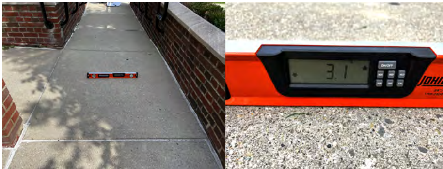
IMAGES 4.1.28 - RAMP LANDING SLOPE 3.1% > 2%
