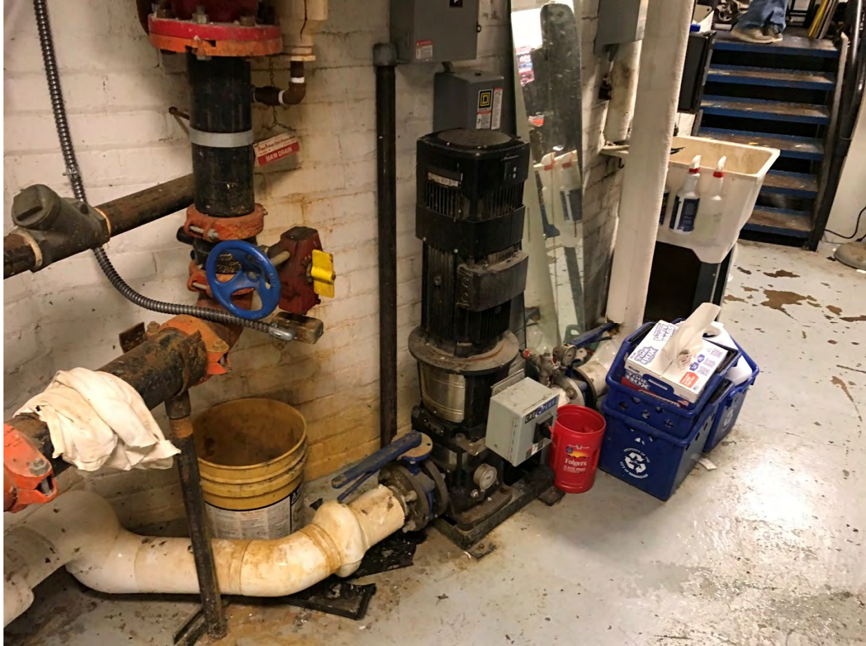
IMAGE 6.18 - WATER BOOSTER PUMP
