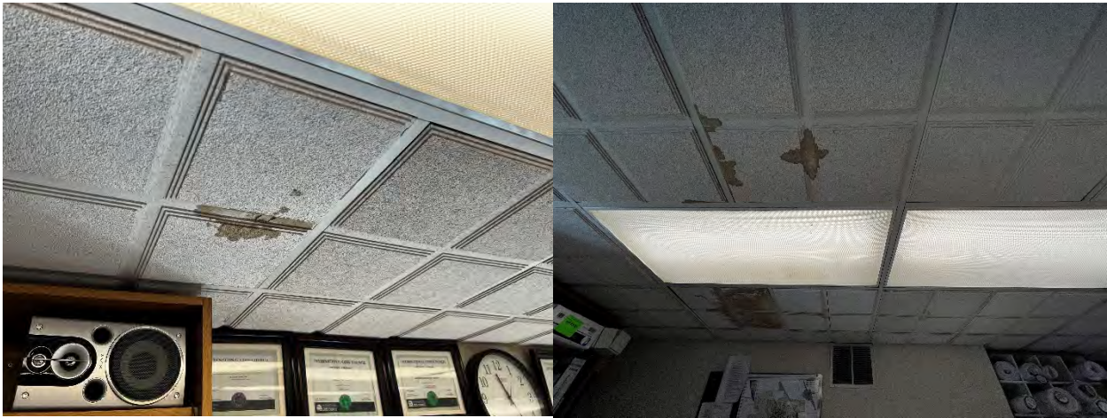
FIGURE 2.3.07 – STAINED CEILING TILES IN THE BUILDING DEPARTMENT.
