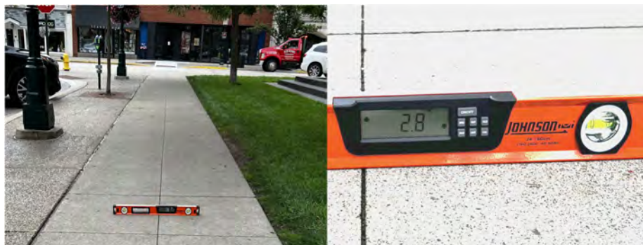
IMAGES 4.1.22 - ACCESSIBLE ROUTE CROSS SLOPE 2.8% > 2%
