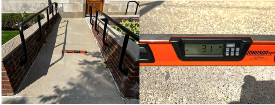
IMAGES 4.1.30 - RAMP CROSS SLOPE 3.1% > 2%
