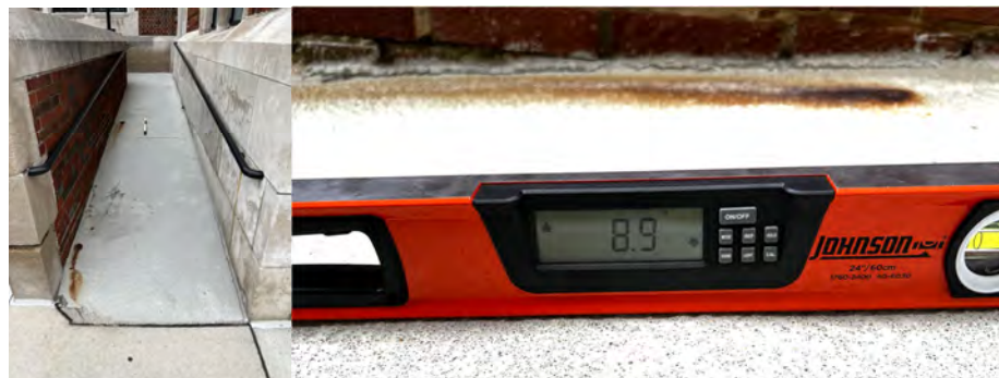
IMAGES 4.1.37 - RAMP SLOPE 8.9% > 8.3%
