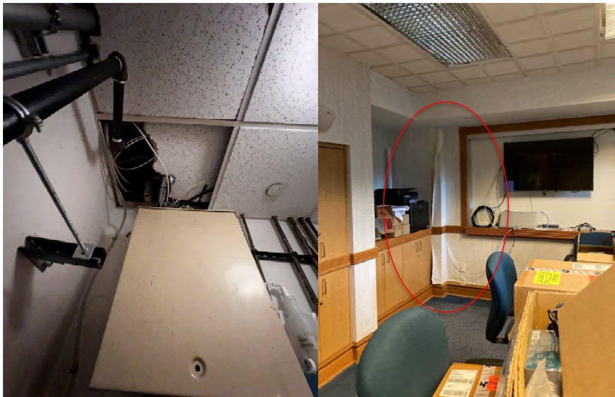
FIGURE 2.3.08 – BROKEN CEILING TILES FOR PIPE PENETRATIONS.
