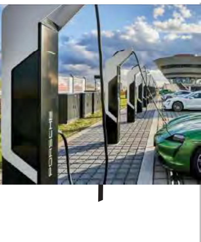
CHARGING STATION (AC) 2 Public Accessible located on Haynes Street
