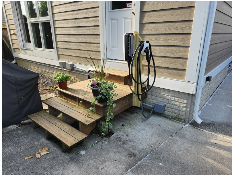
Existing rear landing and EV charger. Structure has deteriorated, is not level, includes no railing. Orientation results in snow drift accumulation against door and step in wintertime, and EV charger is exposed to the elements.
