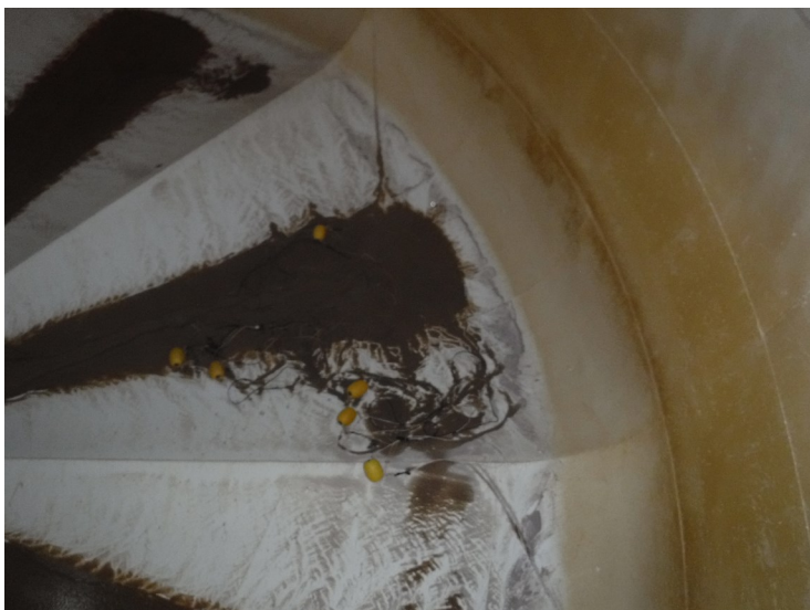
45) Broken ropes supporting the cathodic protection system.
