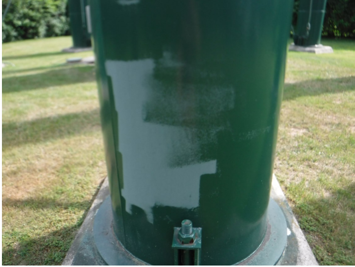
13) Clear coat failures at a leg section.
