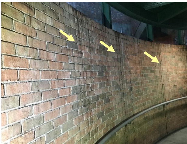
Figure 9. Water tracking down inboard surface of brick.
