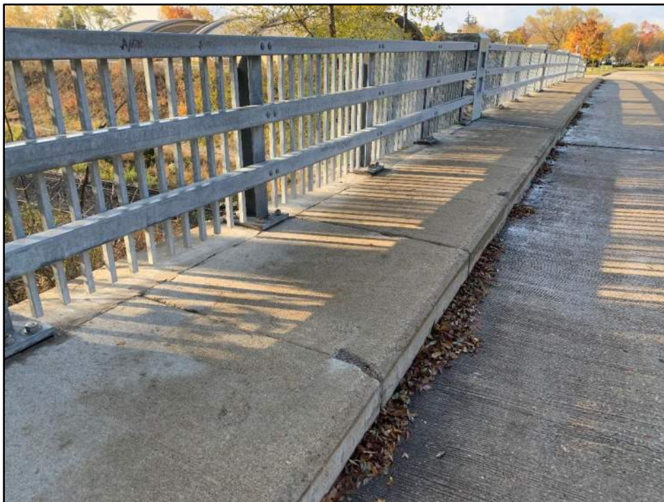
Spalling of south sidewalk
