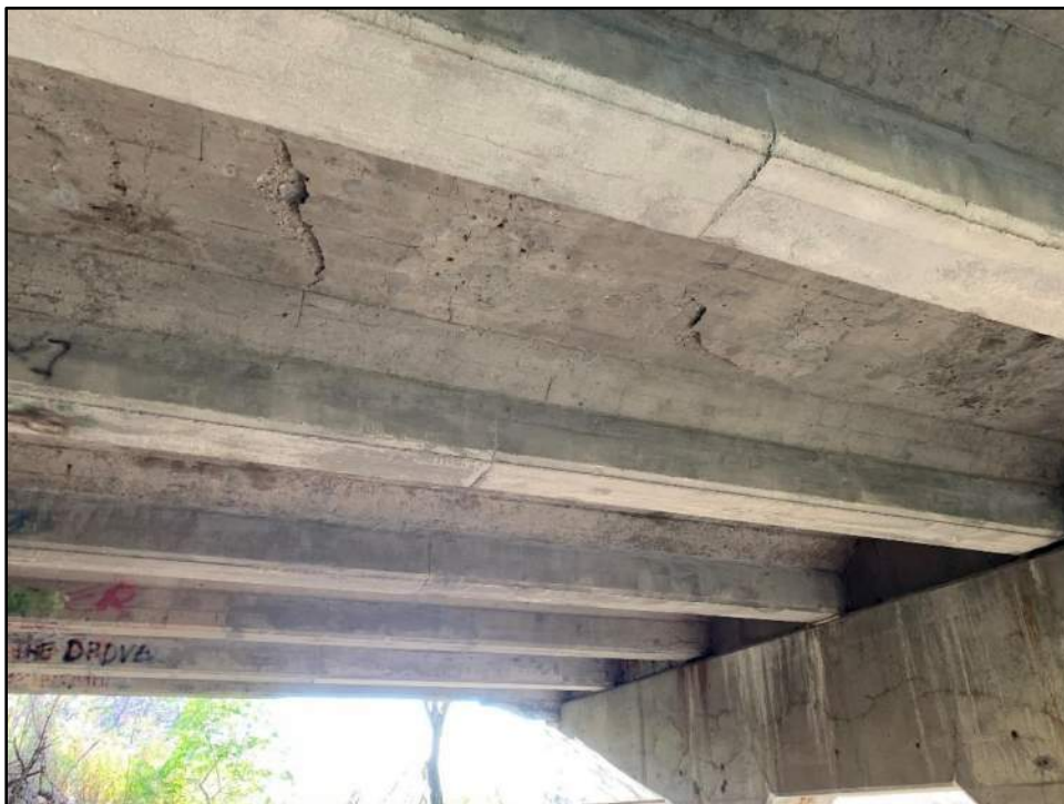
Deck delamination in east span
