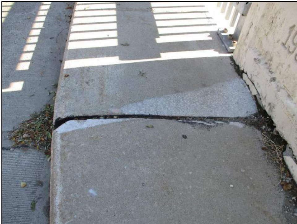
Sidewalk deterioration at abutment
