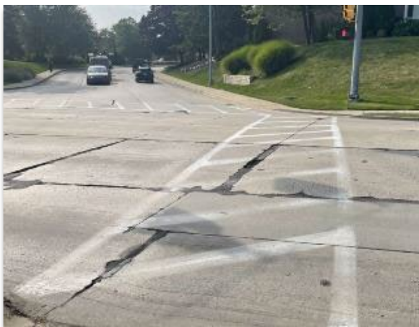
Cracks in the Pavement Along Crosswalks
