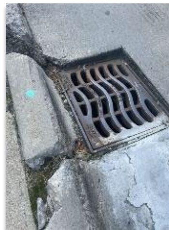
Sunken Drainage Gate at S Eton Street
