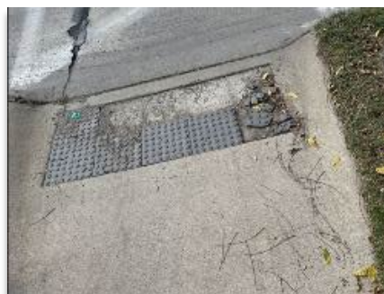
Broken Detectable Warning Pad
